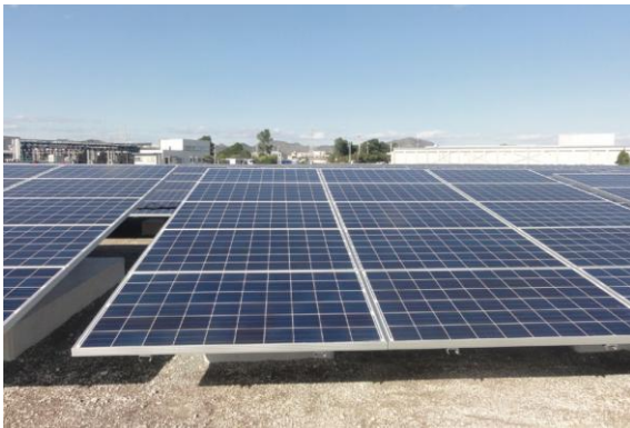
▲Solar panels at the Iho Site, Japan
